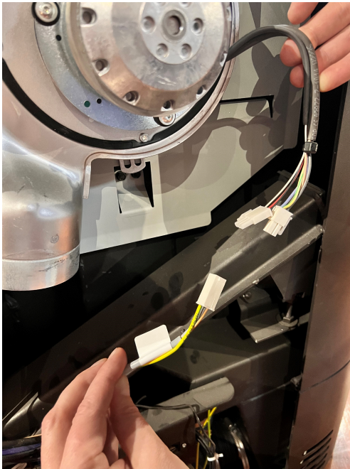
Fig. 7: Connecting the cables
