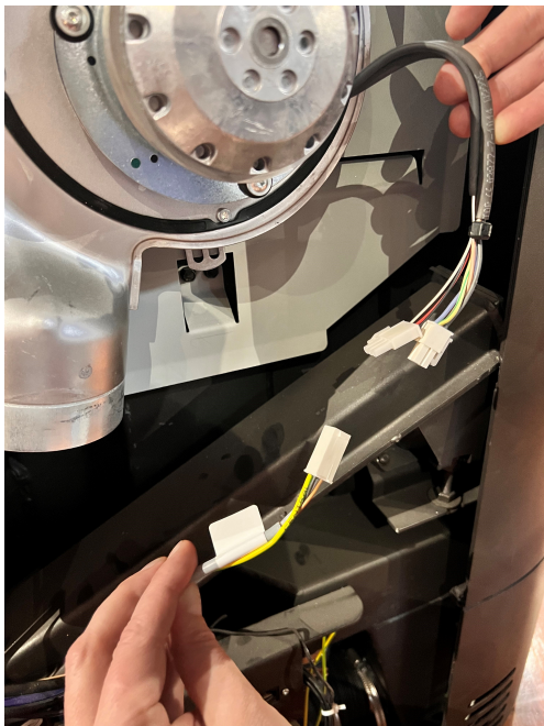
Fig. 22: Connecting the cables
